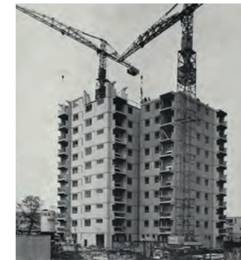
A three storey block and the central tower under construction, both using the Reema Hollow Panel System
