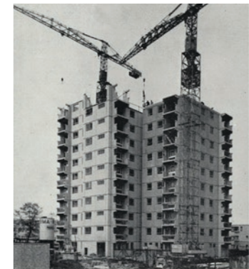
A three storey block and the central tower under construction, both using the Reema Hollow Panel System
